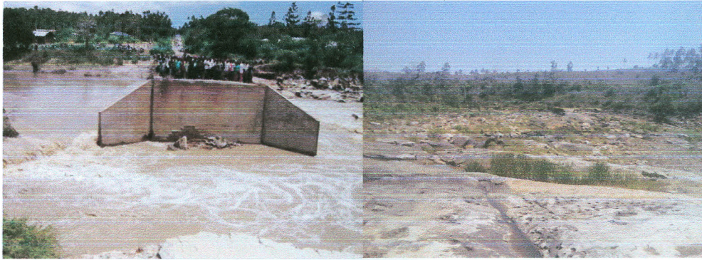
Figure 4-13 Damage to infrastructure Kombeni river Mazera/Kaloleni Road 2006 the same river in dry season
