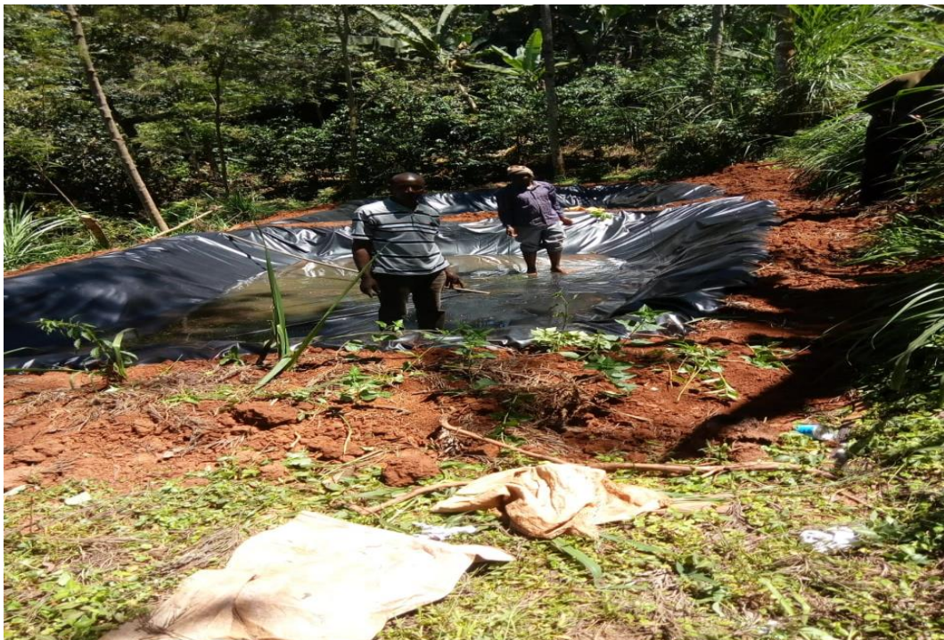
Photograph 3.2: Polythene liners being spread around the fish ponds at Kianjogu in Mathira west sub-county
