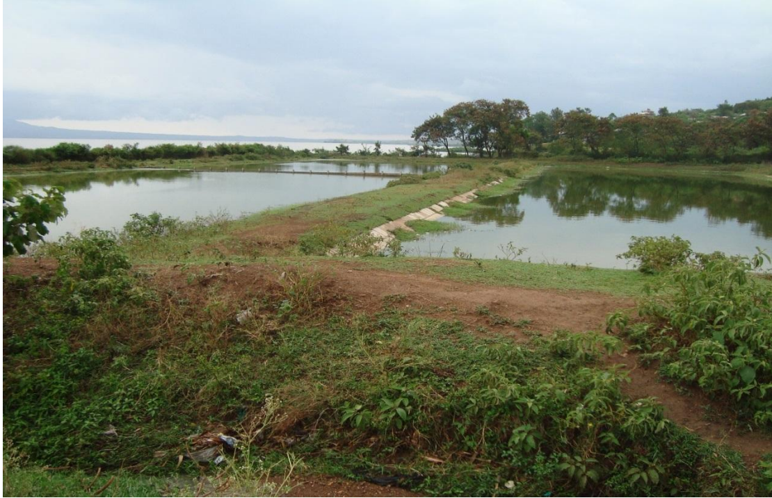
Plate 3.6: Two stabilization ponds of the dilapidated sewage treatment system located near the lake and site L5.
